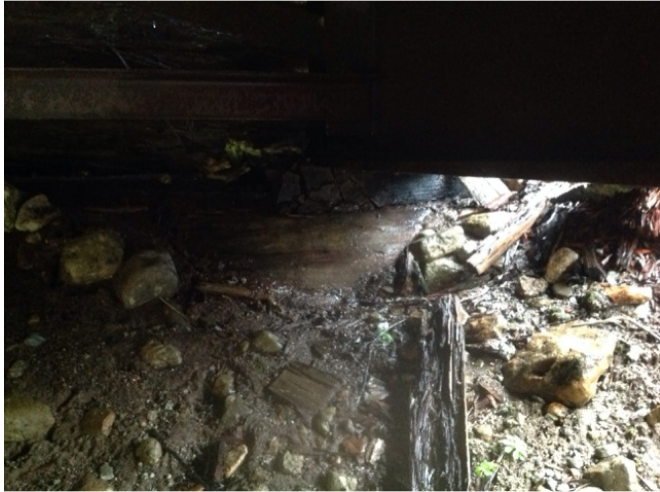
lefty bank timber planks crushing on sill
